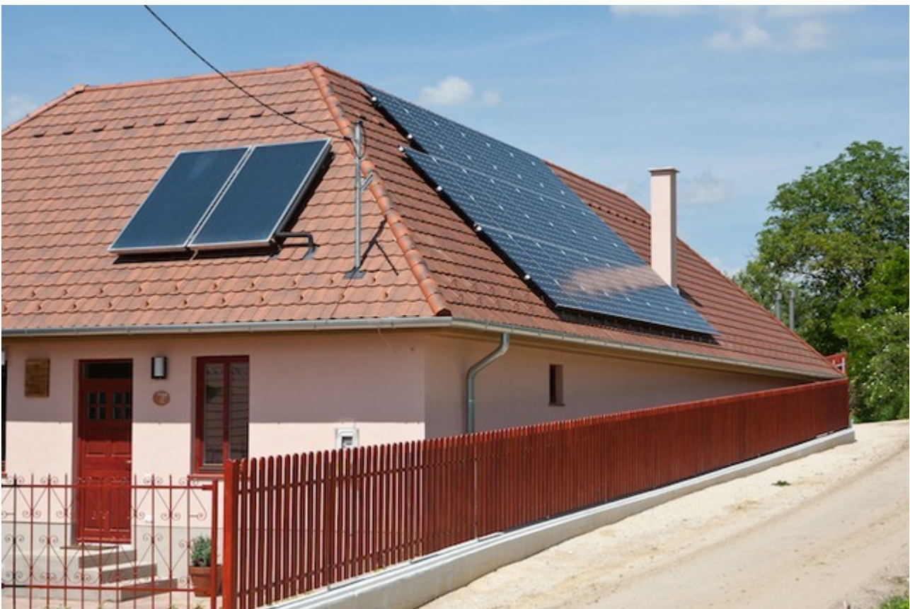
Picture 3: 6.56 kWp photovoltaic solar system (right) and solar collectors (left) at Irota EcoLodge Middle House.
